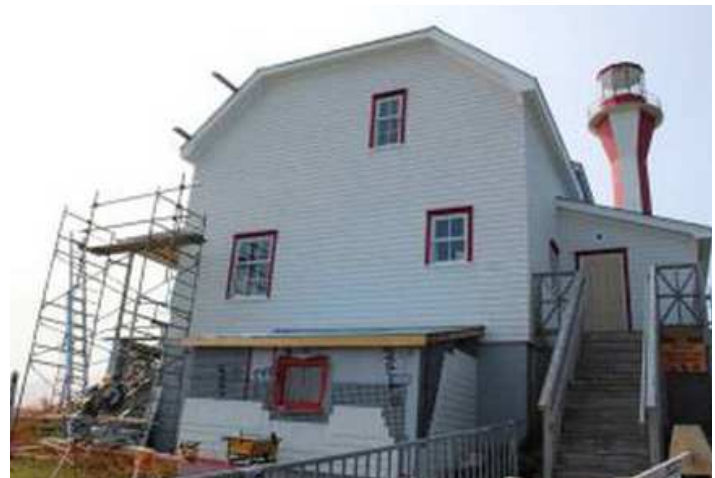
Photo: Allen, Carla. "Yarmouth's Cape Forchu Lighthouse Renovations Nearing Completion." SaltWire, 22 Aug. 2017, www.saltwire.com/business/yarmouths-cape-forchu-lighthouse-renovations-nearing-completion-114558/?location=yarmouthsouth-west-nova-scotia .
